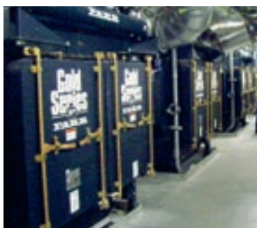
Multiple GS dust collectors on tablet coaters
